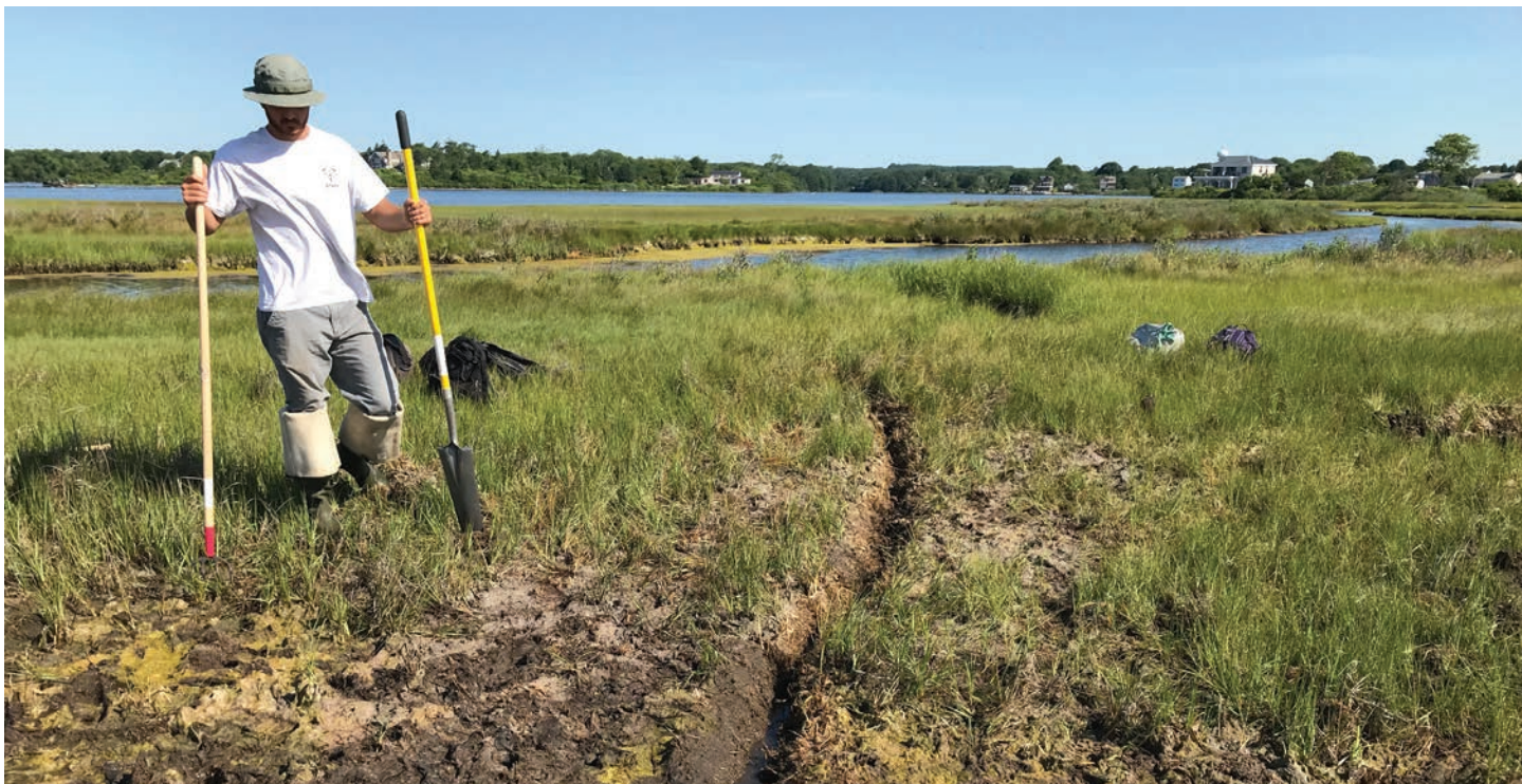
Creating shallow channels, or “runnels,” can reduce ponding and help restore natural hydrology in marsh systems with impaired drainage. Tanner Steves
